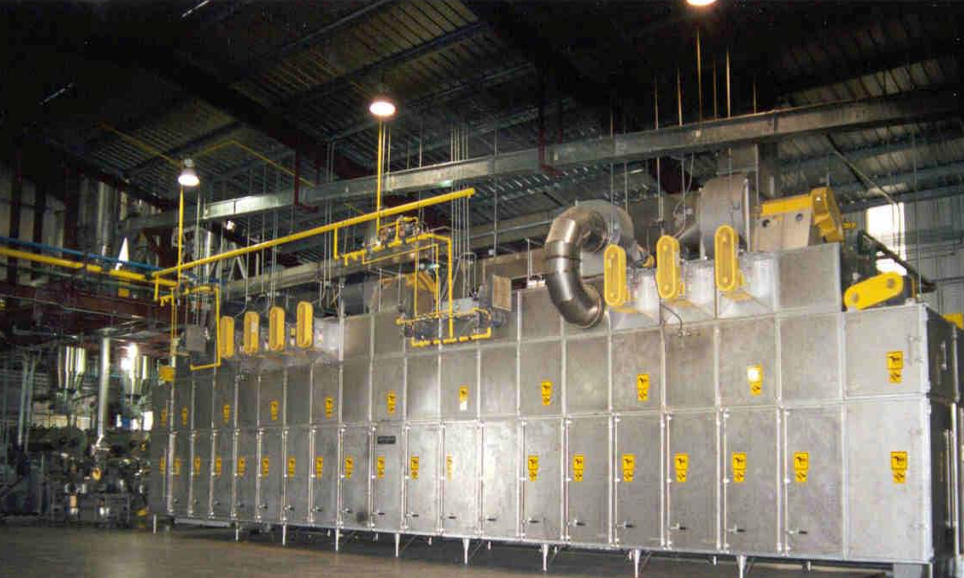
35 ton/hr, 3-pass, fishfeed drier/cooler
